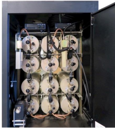
FIGURE 5: PIM TEST EQUIPMENT FOR VHF
